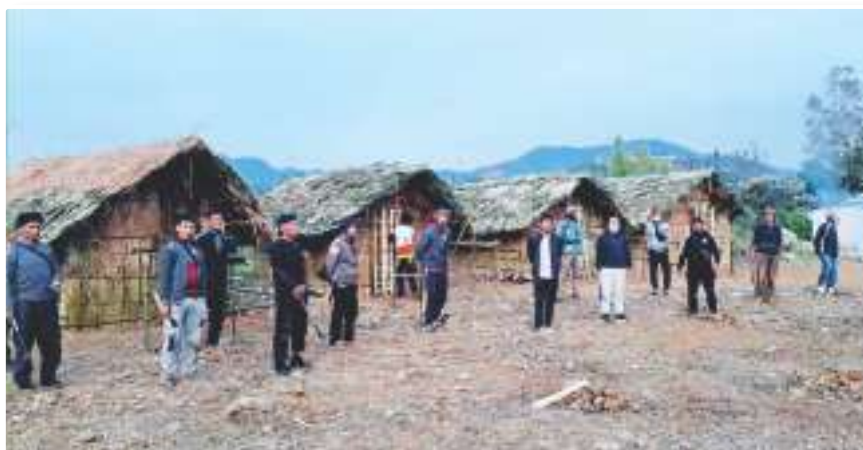
Quarantine House constructed by VLOs with support by Village Council and Student Union
