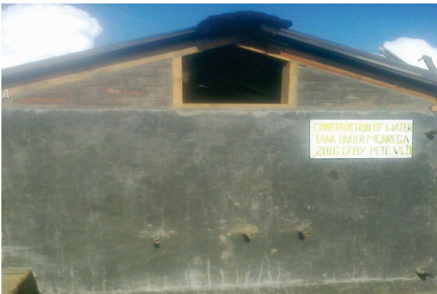
Community water tanks such as this have been constructed in convergence with MGNREGA by VLOs at Khuzama and Kezoma, Jakhama Block, Kohima
